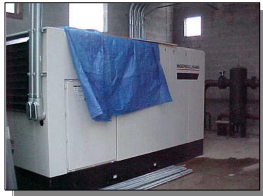
Snow air compressor
